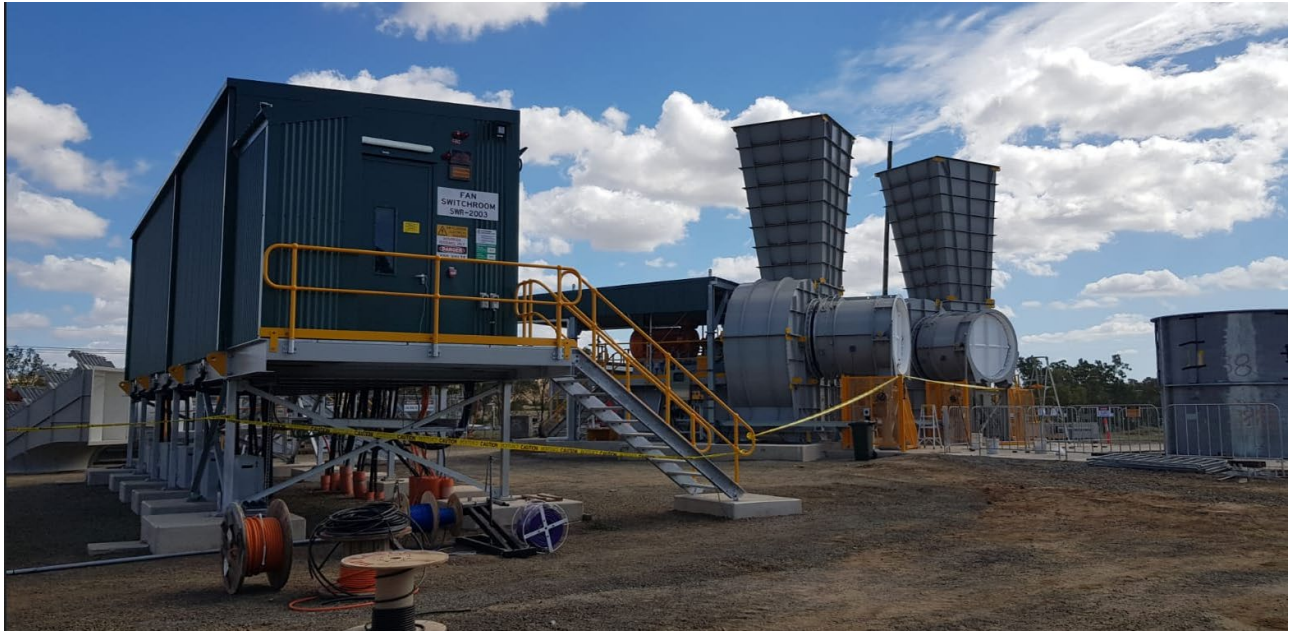
Vent Fan Switchroom FAT, SAT HV Commissioning North QLD ESB Power 2021
