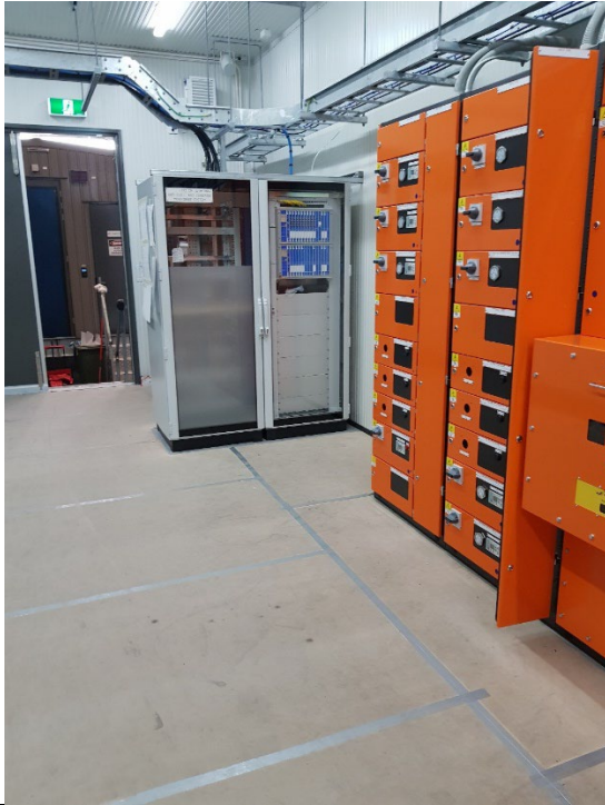
Talinga Gas Train LV Switchroom Roma QLD ESB 2021
